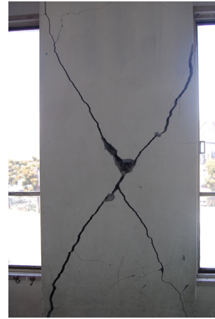
(c) 極短柱のせん断ひび割れ
